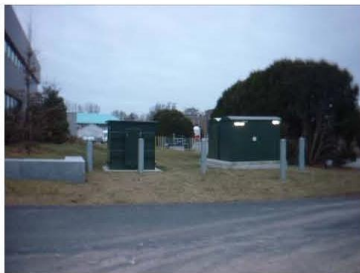
1. Electrical infrastructures: L pad-mounted transformer
