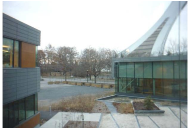
Physical link between the construction site and the existing Biodiversity Centre outdoor garden
